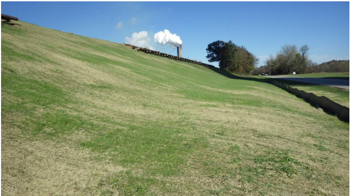
Photograph 8 – New vegetation at possible LVWTS piping crossing on downstream side eastern embankment.
