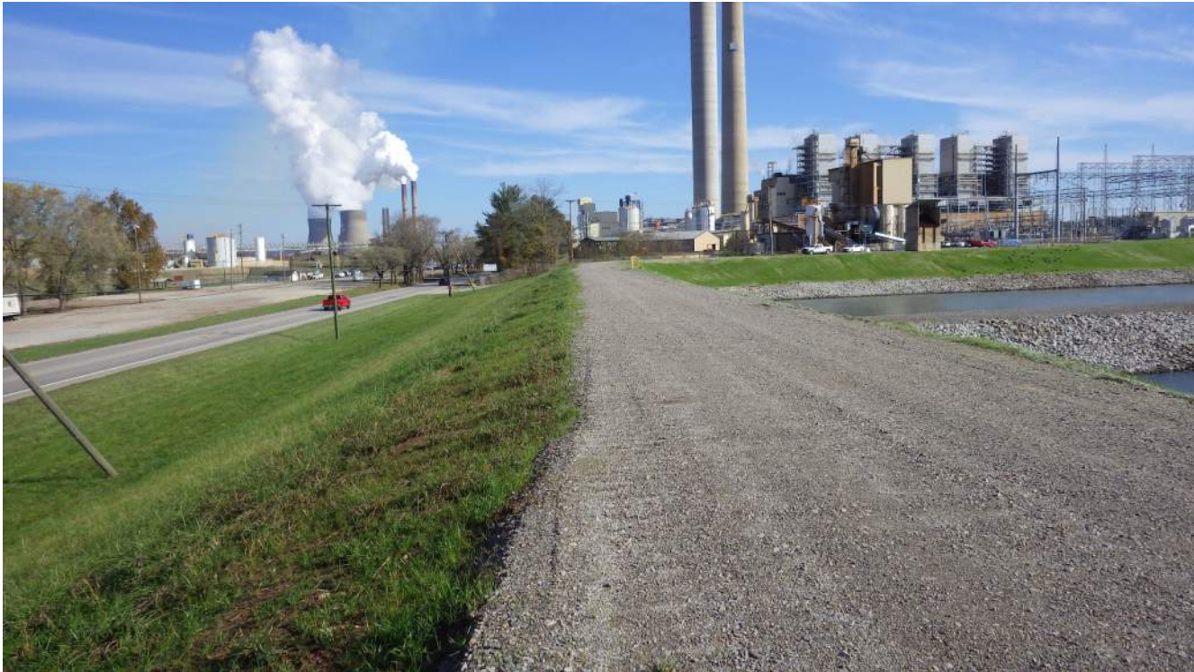
Photograph 5 – Erosion noted at change from access road to grassed slope.
