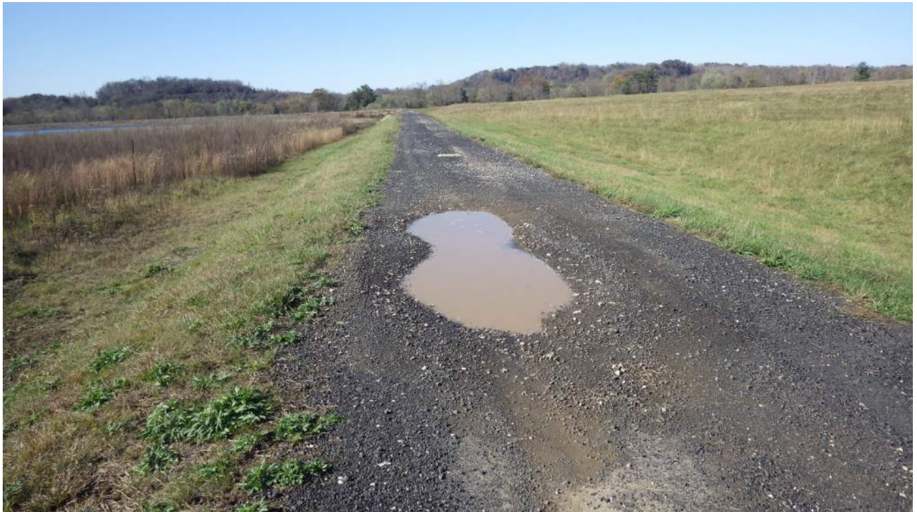
Photograph 10 – Standing water on northern dike.
